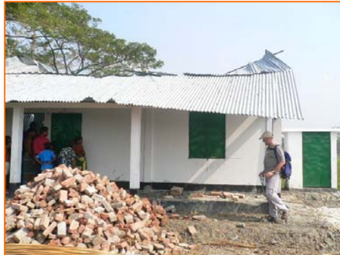
Mr. Ben visited a damaged PRIMA building of Aloshikha on 15 th November 07 after devastating Sidr
